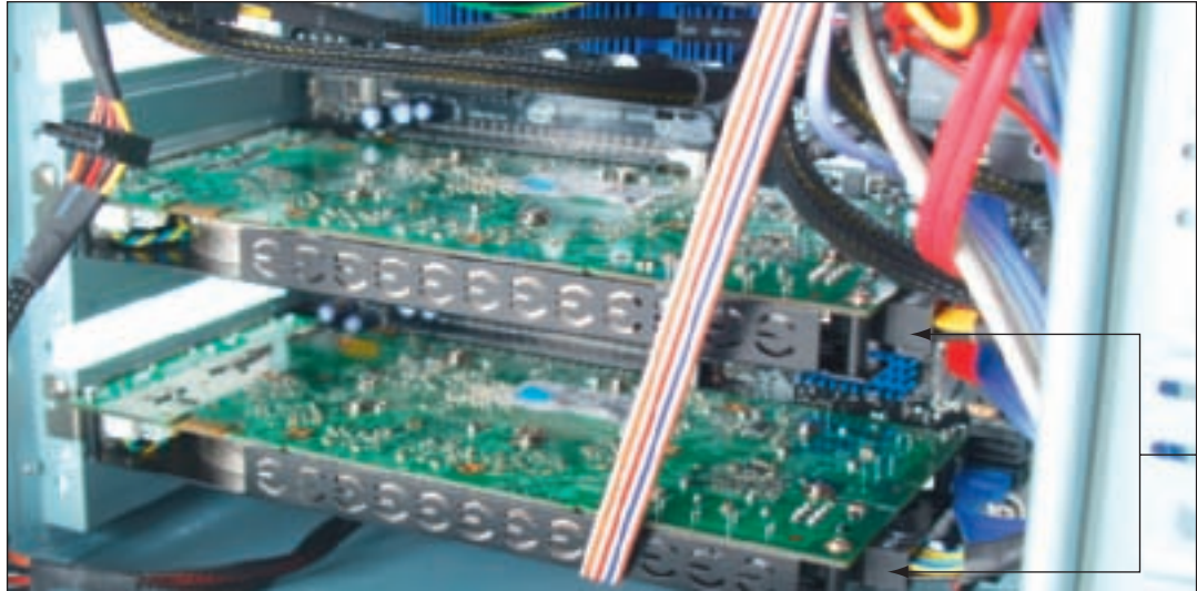
Figure 9-77 Two video cards installed in a system Courtesy: Course Technology/Cengage Learning
