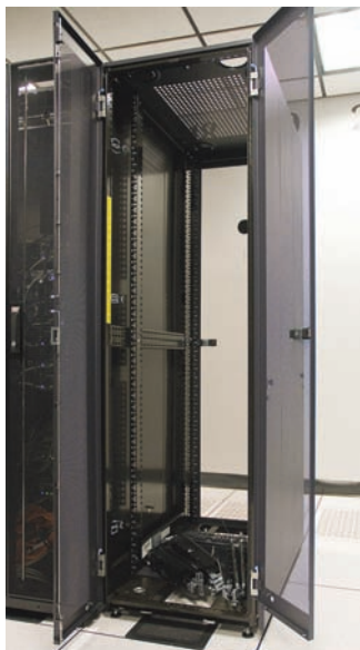
• Figure 22.15 A floor-to-ceiling rack
