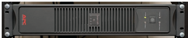
• Figure 22.16 A rack-mounted UPS
